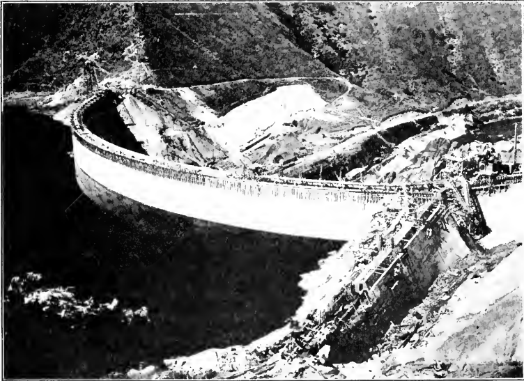
THE ARROW ROCK DAM (Idaho), still building in 1918 when this photo was taken: part of one of the most famous of all the government's projects to irrigate arid lands. This dam is 67 feet higher than the great Roosevelt Dam in Arizona.
